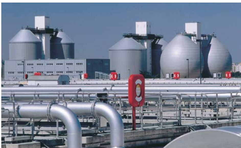
Digestion towers at WWT-plant Wassmannsdorf
