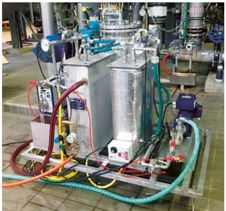
Pilot plant for thermo-chemical hydrolysis at WWT-plant Wassmansdorf
