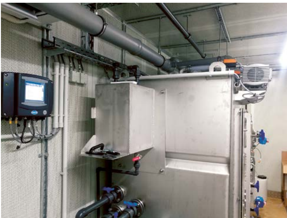
Membrane tank in MBR plant of Martin Systems GmbH
