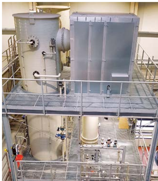
N-recovery system with two units at WWT-plant Brunswick-Steinhof: ammonia stripping unit and ammonia gas scrubber
