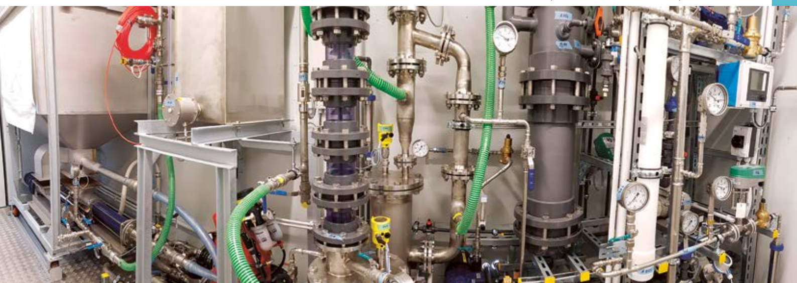
Pilot plant for vacuum degasification and production of ammonium sulphate
