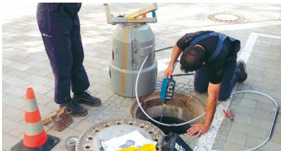
Installation of an automatic sampler
