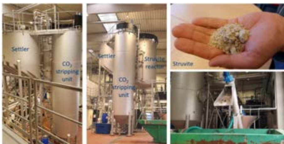
Figure 59 Pictures of the struvite production unit consisting of a CO2 stripping unit, a struvite reactor, a settler and a container to collect the harvested struvite crystals (NuReSys process).
