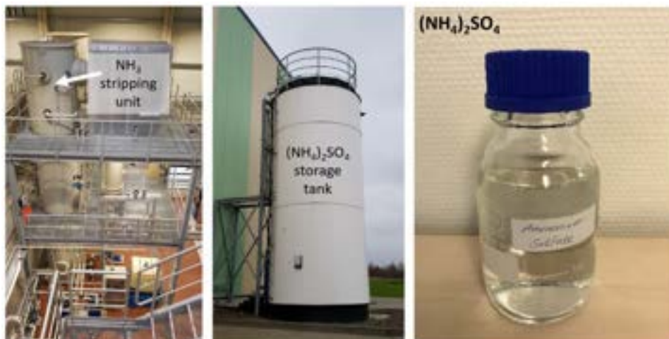
Figure 42 Pictures of the ammonium sulphate production units, the storage tank and an ammonium sulphate solution sample
