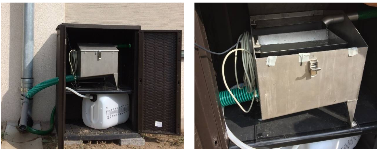
Figure A3. Tipping counter for measurement and sampling of roof runoff.
