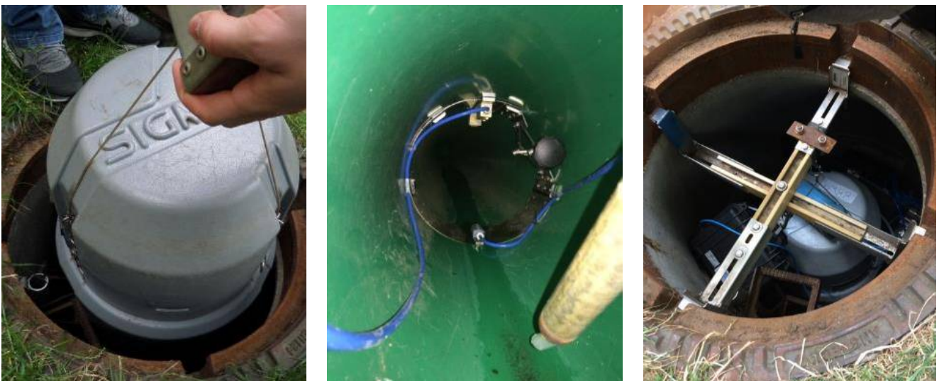
Figure A4. Installation of an automatic sampler and flow measuring device in a storm sewer and a manhole.
