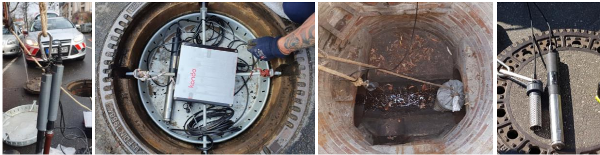
Figure 8: KANDO's smart unit and sensor (left), the EC sensor and logger (right) as well a sensor installed at a sewer manhole (right).
