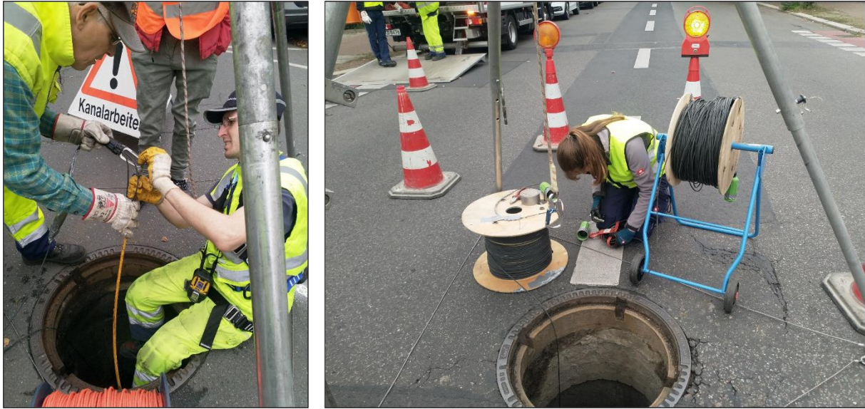
Figure 17: Storm sewer manhole located in the middle of the street (right); preparations to realize access to the sewer system via house connection (left).
