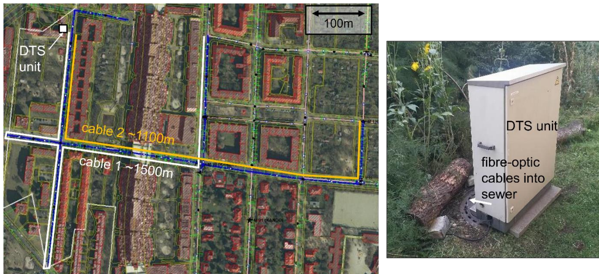
Figure 15: Overview of studied sewer system and fiber-optic cable routes (left); DTS unit installed at Bezirksamt Charlottenburg (right)
