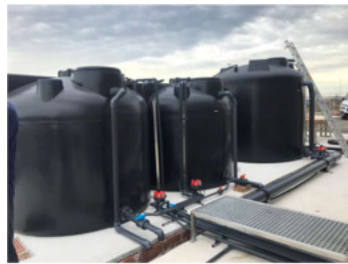
(b) Storage tanks
