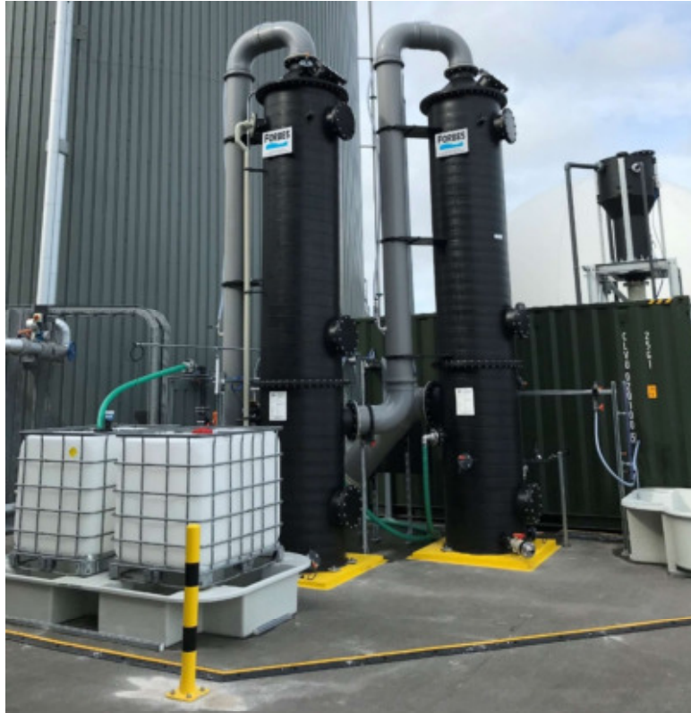
Figure 96. Ammonia stripping/scrubbing unit.
