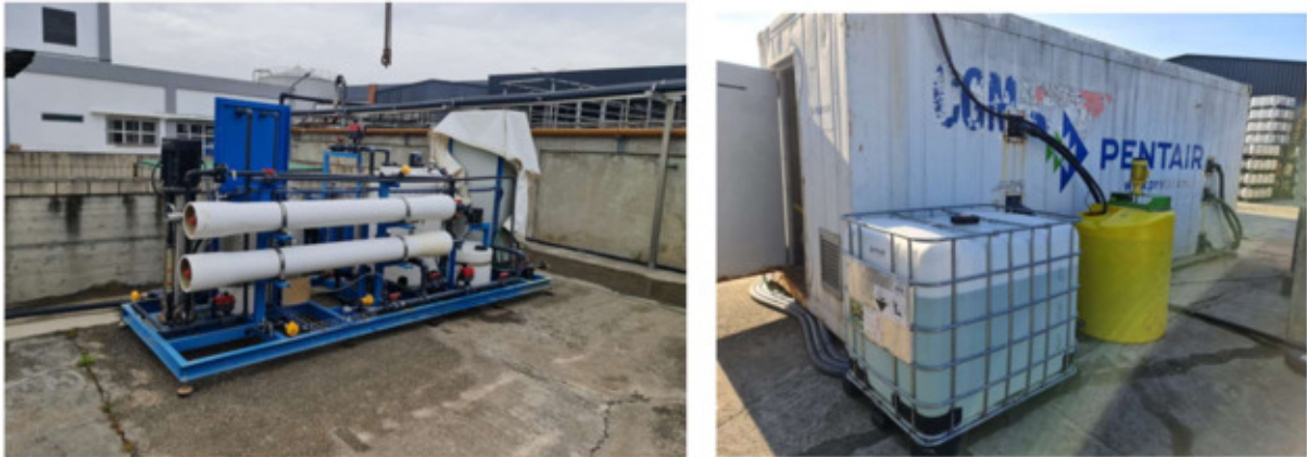
Figure 57. Pictures of RO (left) and NF (right) pilot plants used for the water reclamation case in CS5.
