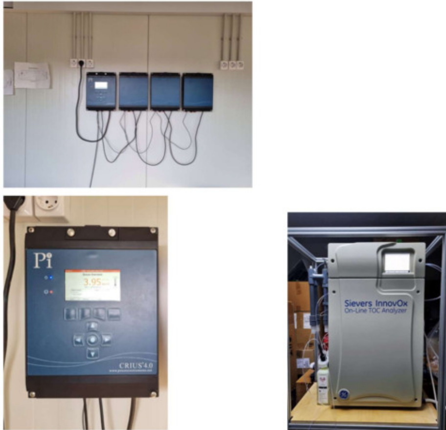
Figure 51. CS4 pilot plant sensors, control unit and TOC analyzer.
