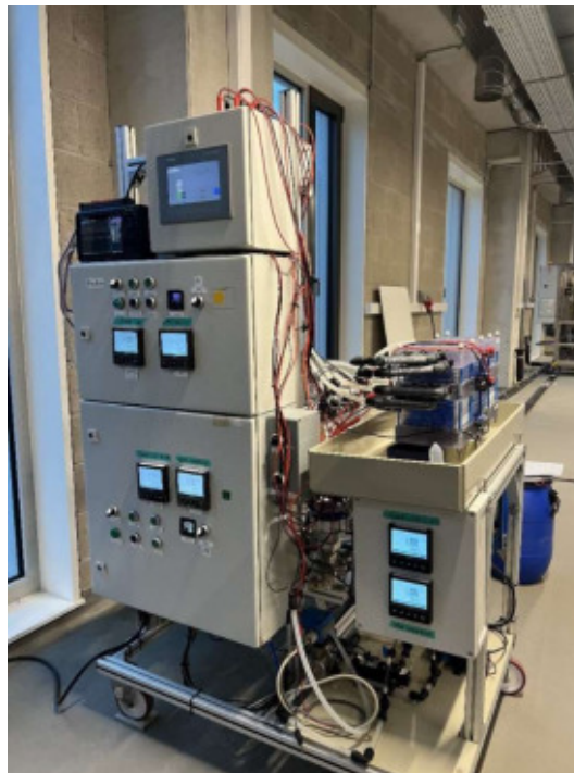
Figure 23. ED pilot installation.
