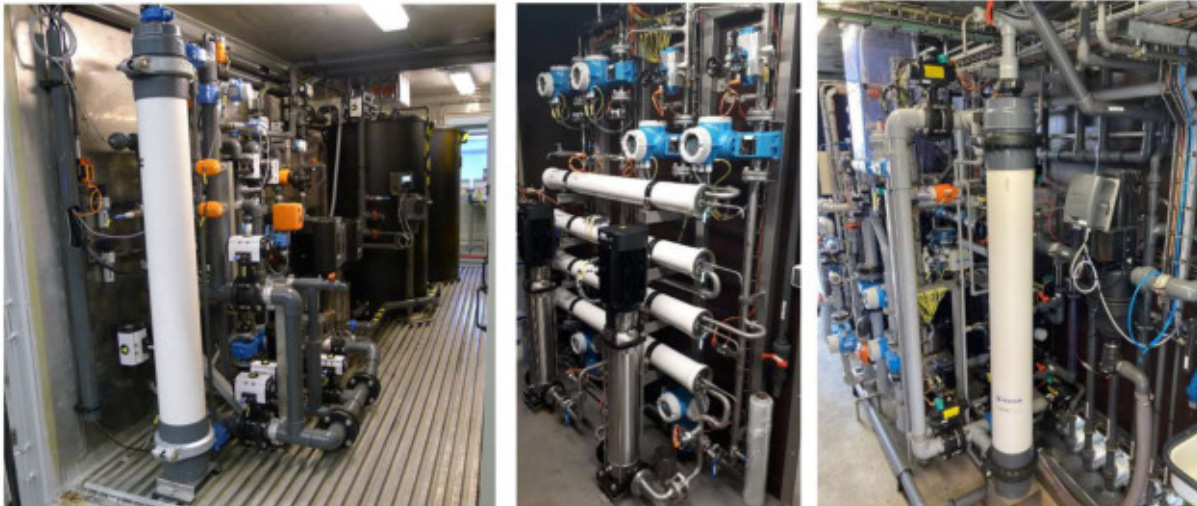
Figure 116. Pilot A - left: conventional ultrafiltration module; Pilot B - middle: reverse osmosis units and right: novel UF/NF module.
