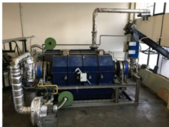
Figure 38. Rotary kiln for slow pyrolysis (PYROCK).
