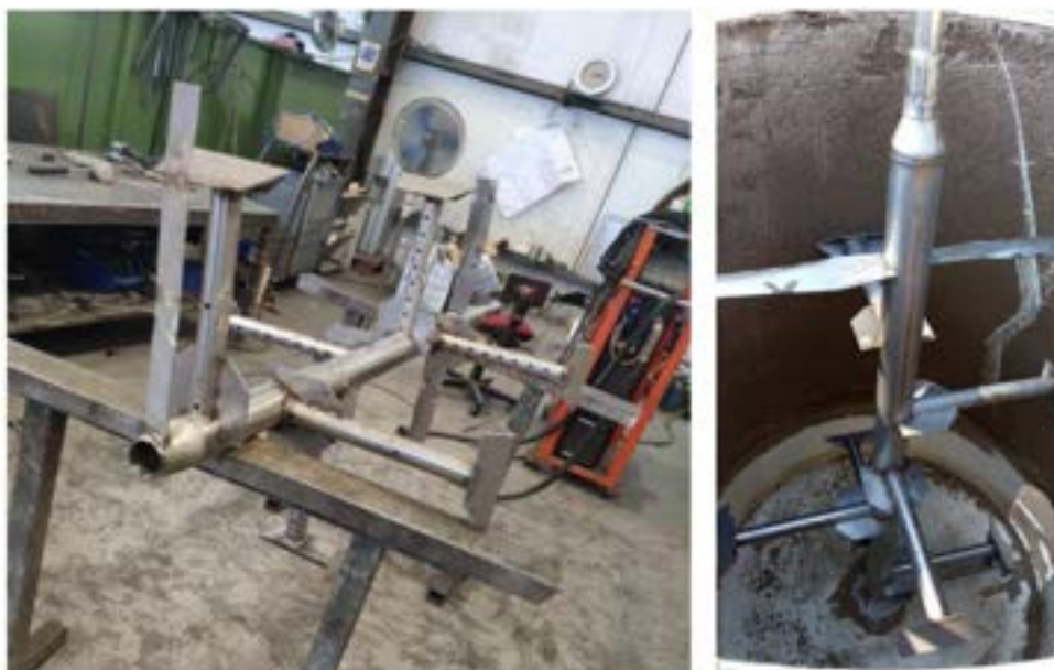
Figure 11 Readjustment of the existing elements of the mixing arm
