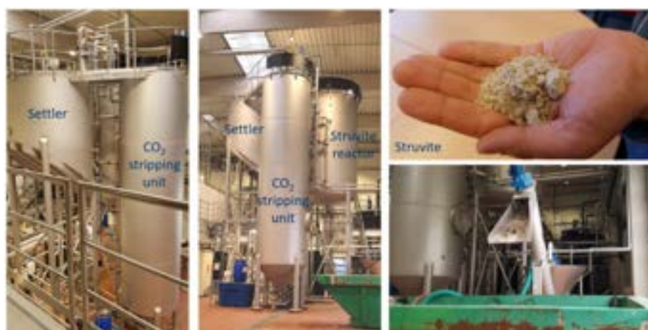
Figure 59 Pictures of the struvite production unit consisting of a CO2 stripping unit, a struvite reactor, a settler and a container to collect the harvested struvite crystals (NuReSys process).
