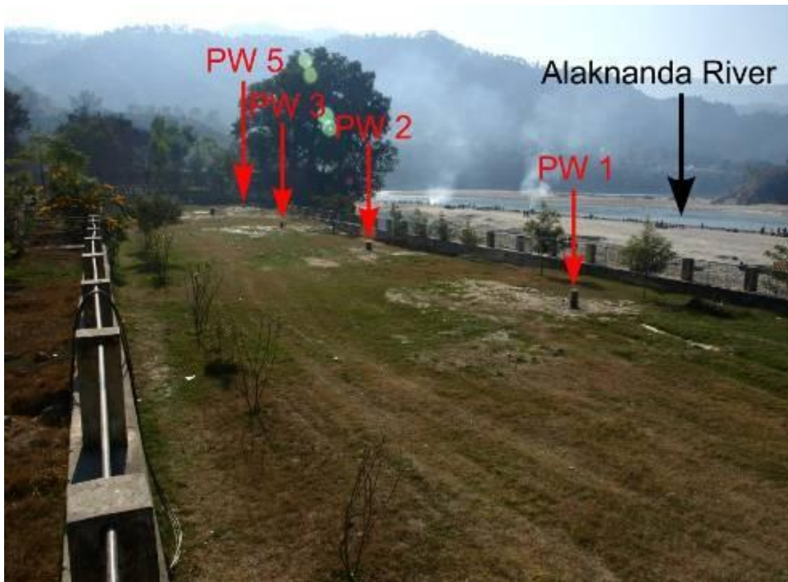
Figure 15 Four additional boreholes for production wells were drilled in July - September 2011 (Photo: F. Musche & E. Ballmann, HTWD, 2011)
