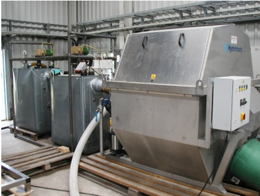
Figure 1: Pilot plant for preliminary tests (May 2009)
