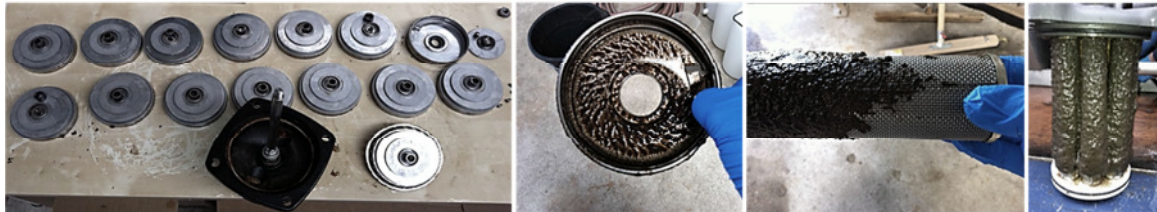
Figure 56: Cleaning of the backwash pump and the strainer of the backwash system
