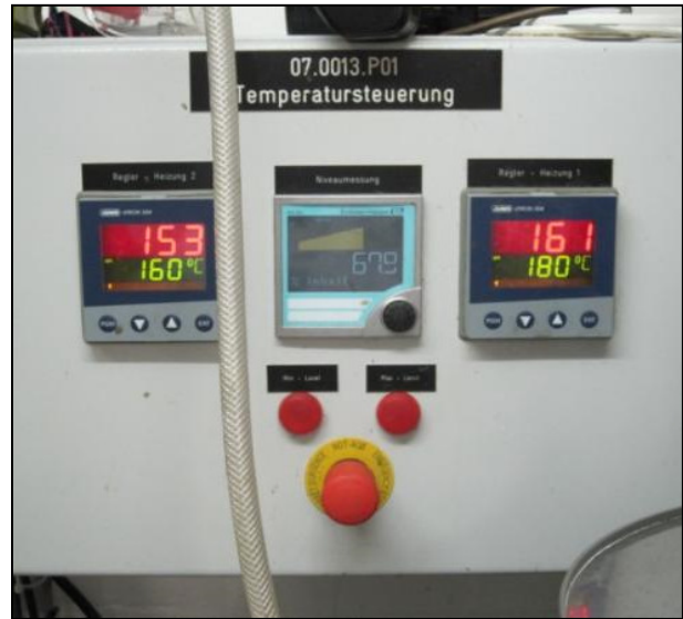
Figure 2-5: Control unit of the THP.
