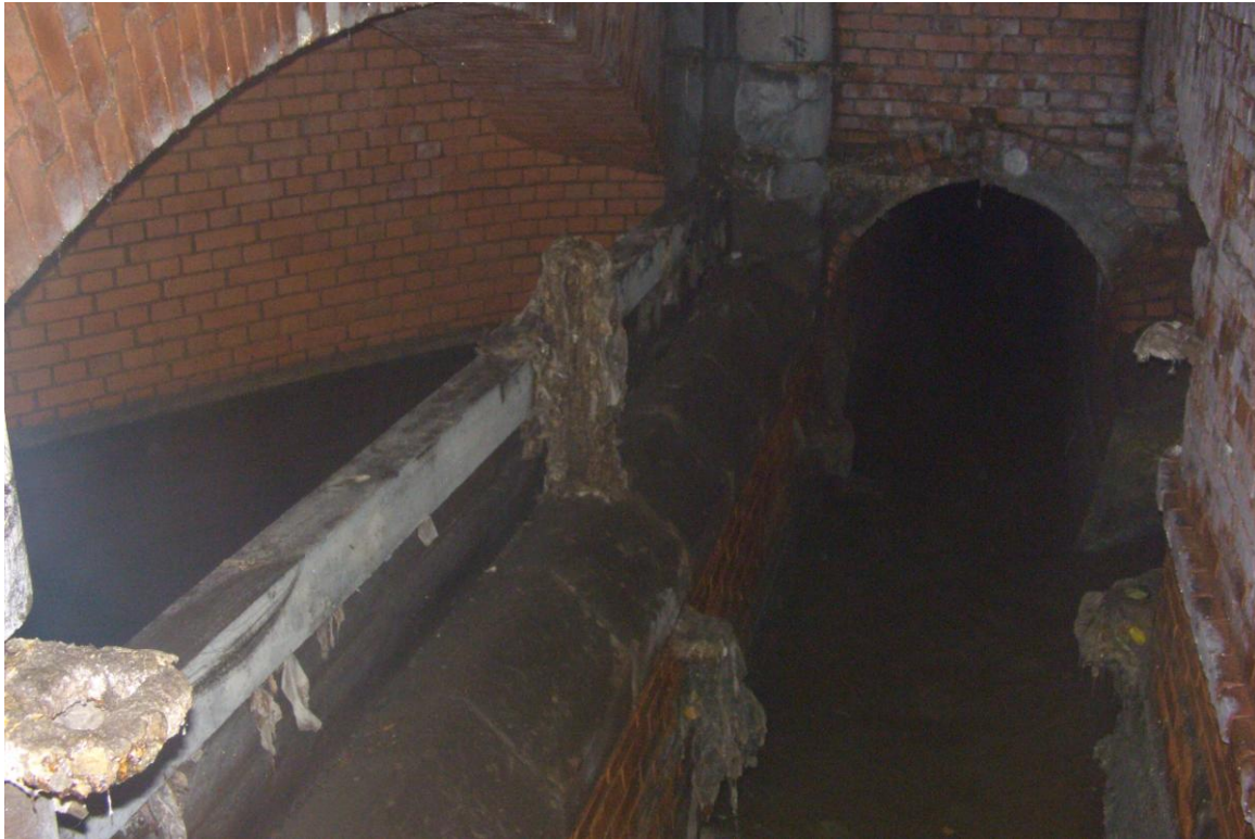
Figure 3. This picture shows the main CSO outlet discharging in the monitored overflow sewer. On the right side of the picture flows wastewater in the combined sewer system. The overflow threshold is composed of two parts: a first level of brick and 40 cm at the top of wood. The wood part was removed at the beginning of 2011 to decrease the CSO threshold.
