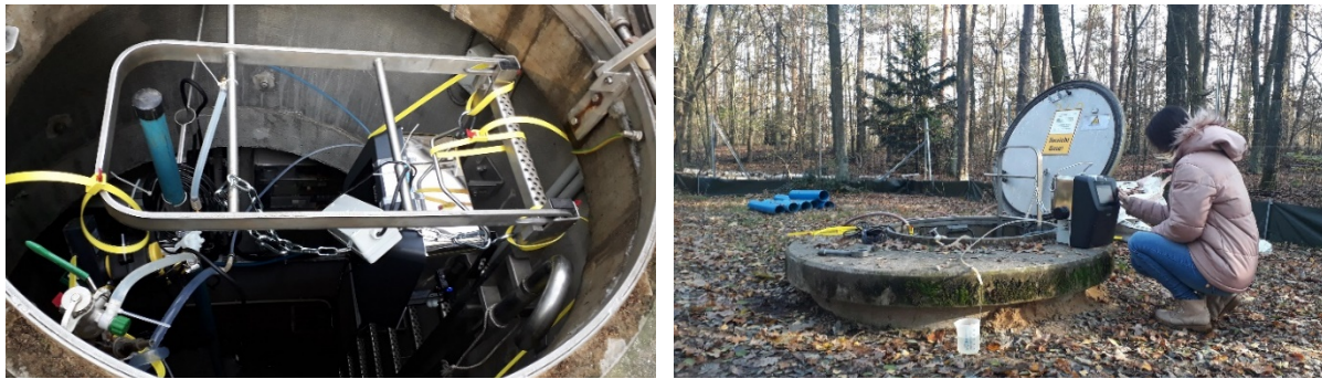
Figure 9. Flow cytometer installed in well chamber (left); flow cytometer maintenance and manual measurements (right)
