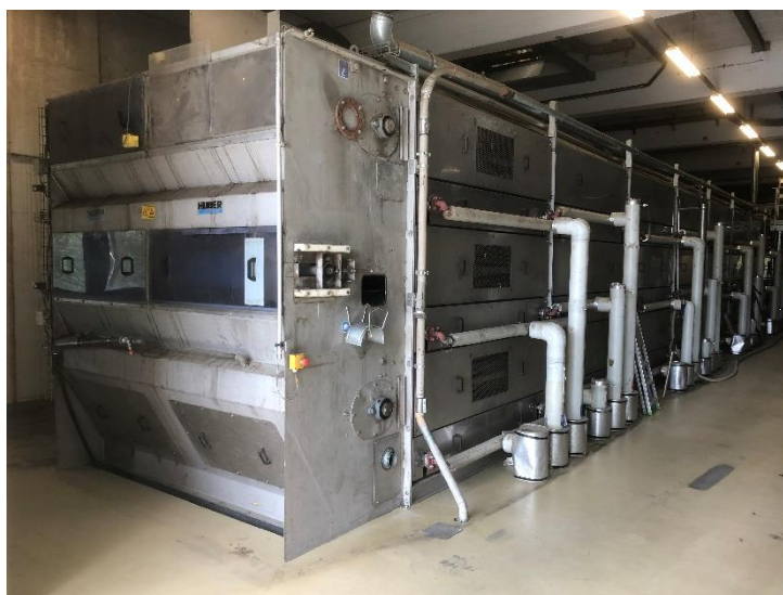
Figure 1. Picture of the drying unit of the sludge treatment stage
