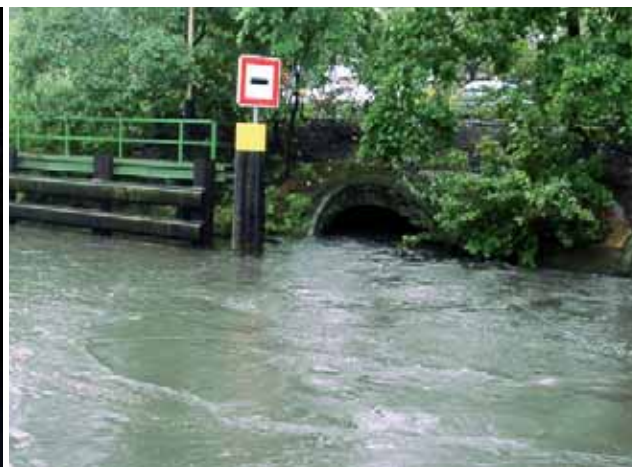
CSO discharge into receiving river
