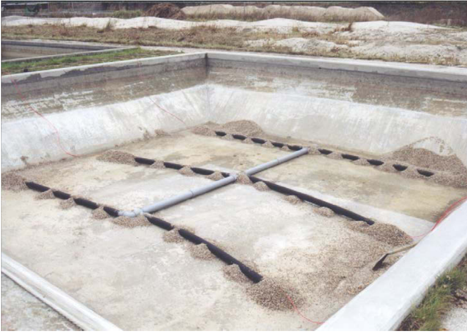
Figure 36: Drainage pipes on the basis of the slow sand filter during sand exchange.
